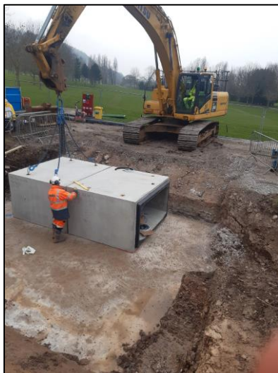
Left: Installation of a 6.5T box culvert units to form the new vehicular bridge at Abergele Golf Club
