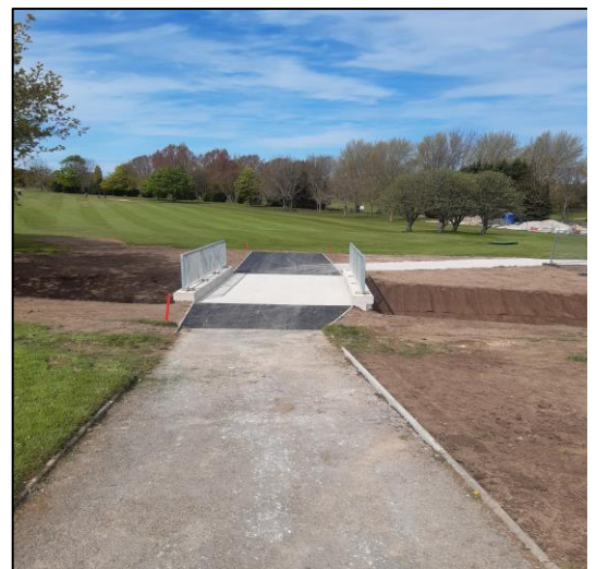
Right Completed vehicular bridge access at Abergele Golf Club, leading from the first tee.
